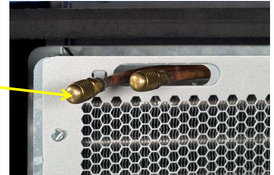
Air Bleed Valves
