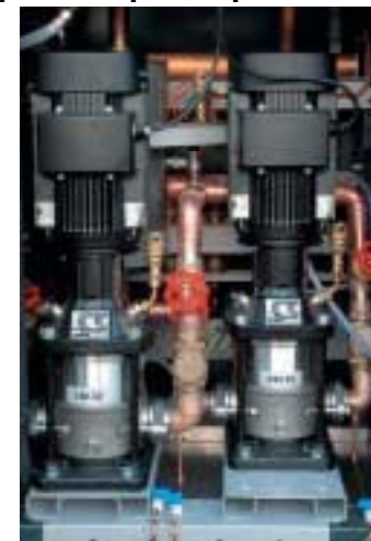
Redundant variable speed pumps
